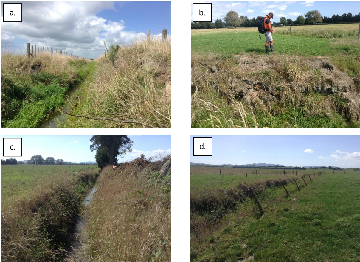
Figure 5: Figure 5a and 5c indicate the typical channel form along reaches 9 and 10 respectively. Figure 5b and 5d illustrate upper bank instabilities along reaches 9 and 10 caused by steep bank angles and poor fence alignment.
